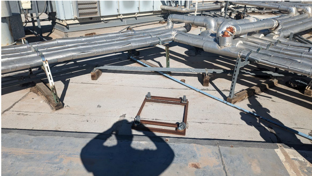
4. Rotten or damaged wood sleepers will be replaced as part of the base bid.
