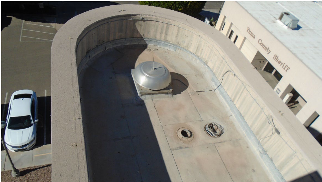
2. There are two small, slightly lower roof areas that are included in Building F.
