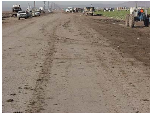
Example of unsafe use of roadways and a need for clean-up from agricultural activities.
